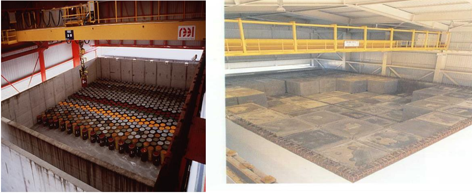
Figure 8-6. Filling and grouting of waste compartments at CSA and El Cabril. (Courtesy of Andra and Enresa)
