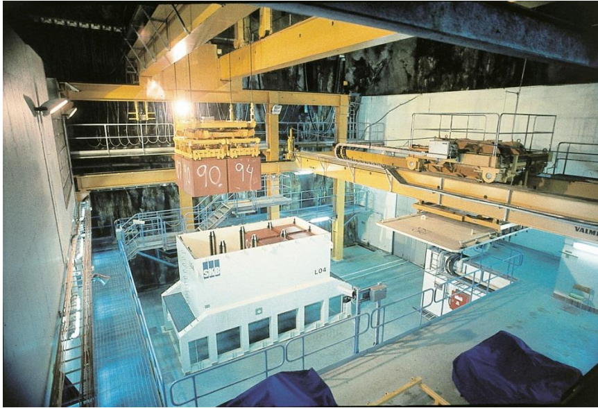
Figure 7-6. Remote unloading of a shielded transport container in the SFR repository in Sweden.
